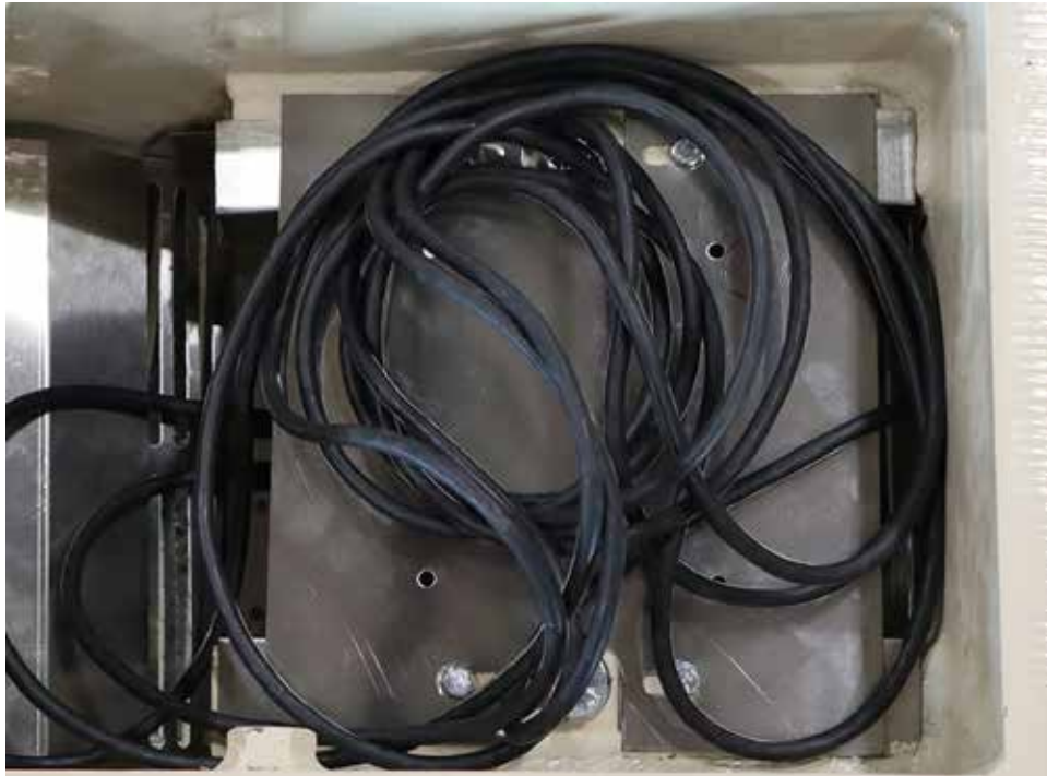
Figure No. 13 – Coil excess cable and place on the stainless steel cable tray.
