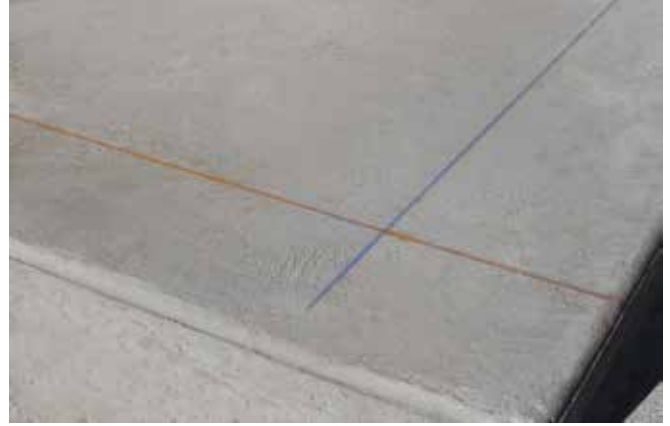
Per foundation drawing, snap a lateral chalk line for aligning load cell stands.
