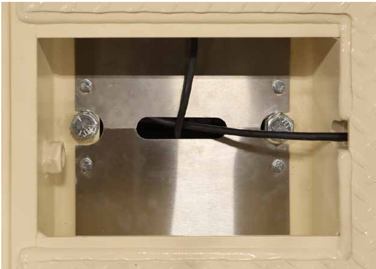
Installed Rodent Guard for 12-Inch Steel Beam Deck Shown
