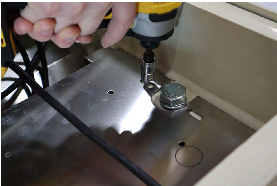
Figure No. 10 – Place the stainless steel cable tray under the cables in the load cell pocket.
