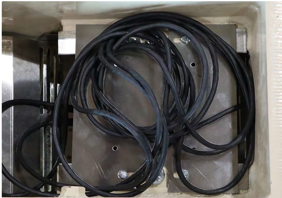
Figure No. 12 – Coil excess cable and place on the stainless steel cable tray.
