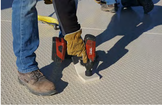
Remove the lifting lugs from the first bridge and install them on the second.
