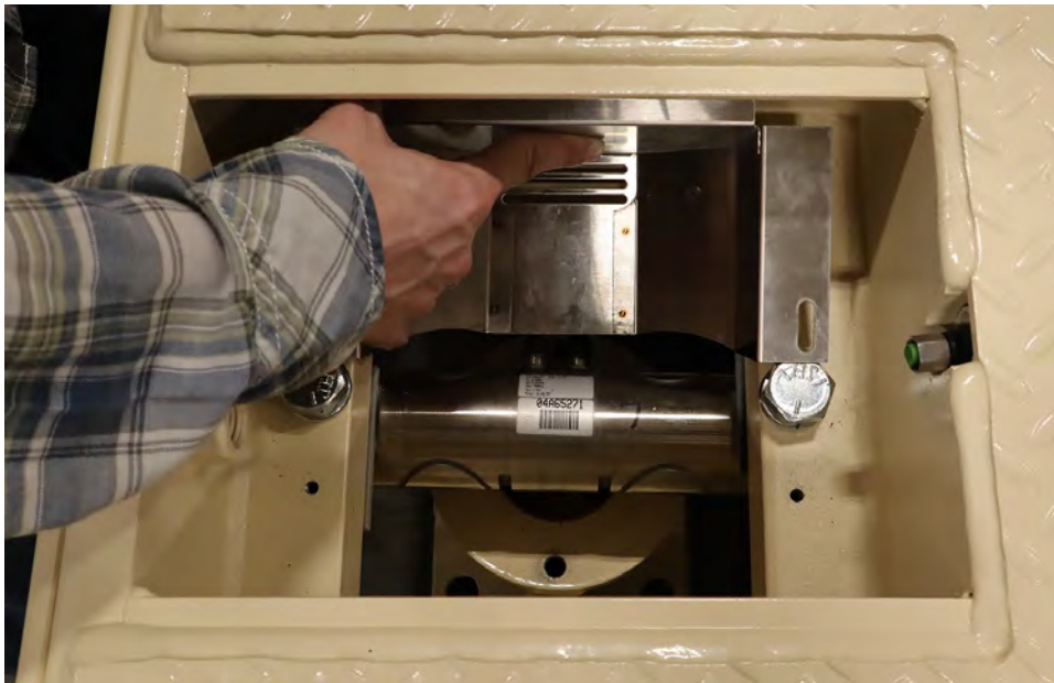
Figure No. 2 – Tilt load cell guard at an angle and slide under load cell cable connectors.
