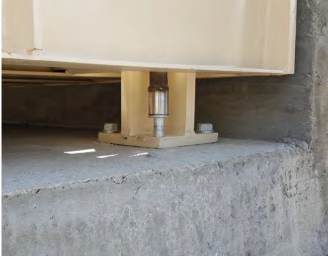
Insert anchor bolts and use a 1 1/8-inch socket and impact wrench to tighten.
