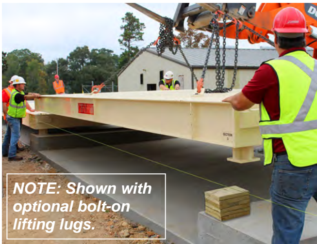
Lower second bridge onto wood blocks and support blocks of the first bridge.
