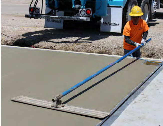
Before concrete becomes non-plastic, deck surface should be further finished to provide a uniform surface texture.
