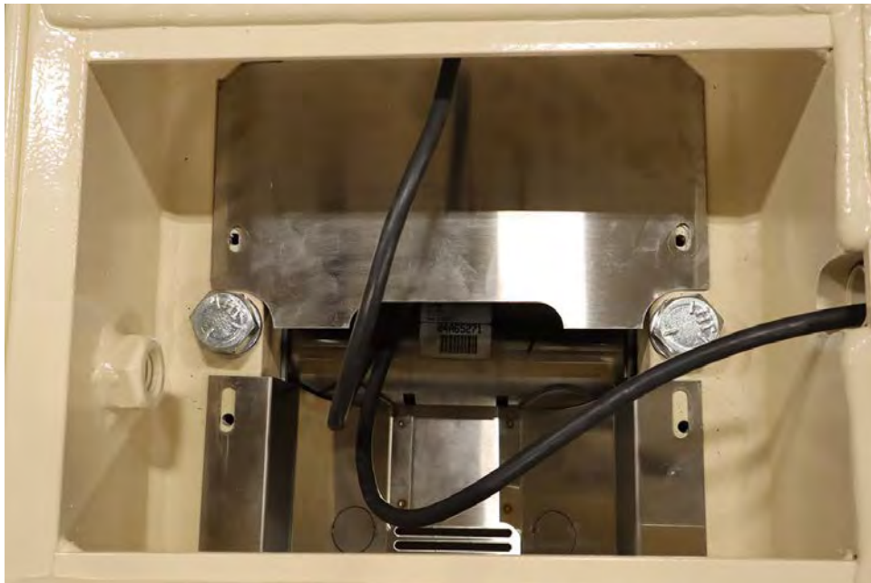
Figure No. 8 – First load cell guard cover installed and positioned over threaded holes.
