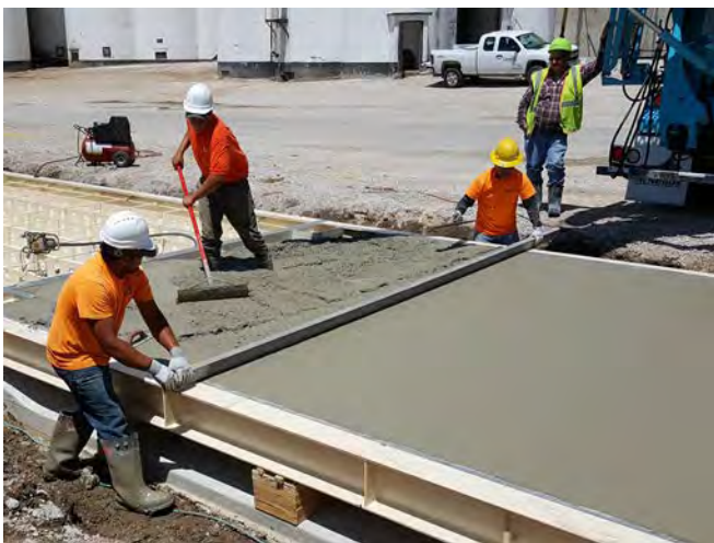
The screed must retain shape and span the lateral width of the deck.
