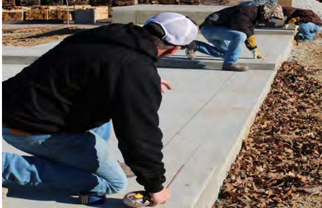
Snap a longitudinal chalk line on edge of piers per foundation drawing.
