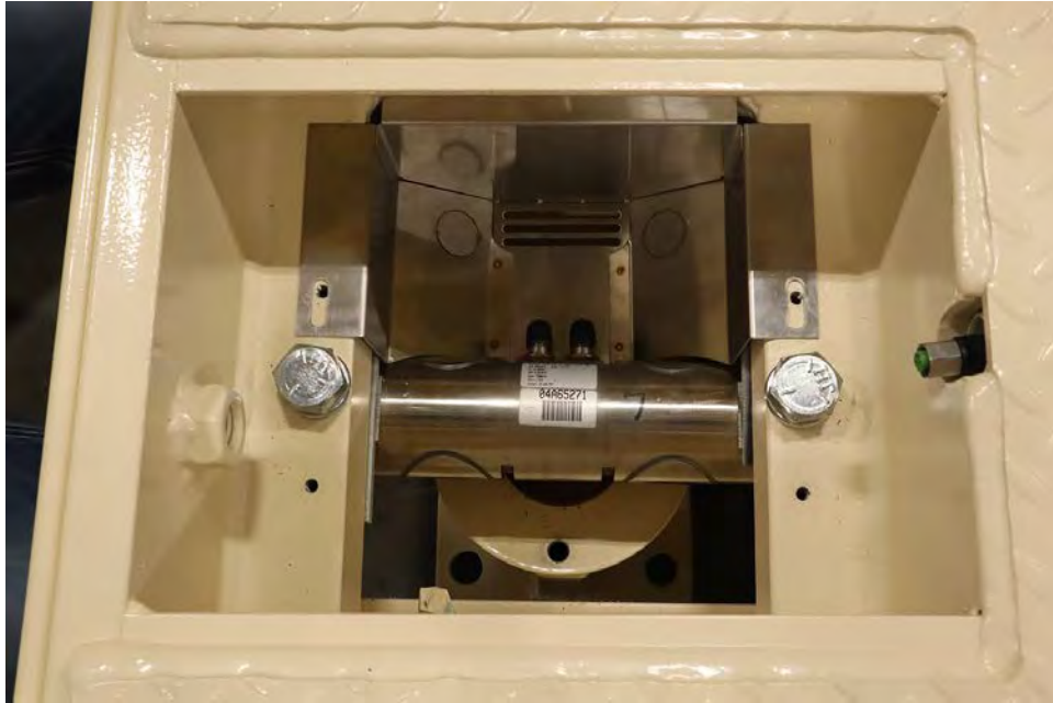
Figure No. 3 – First load cell guard installed and positioned over threaded holes.
