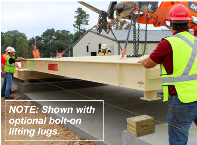
Lower second bridge onto wood blocks and support blocks of the first bridge.
