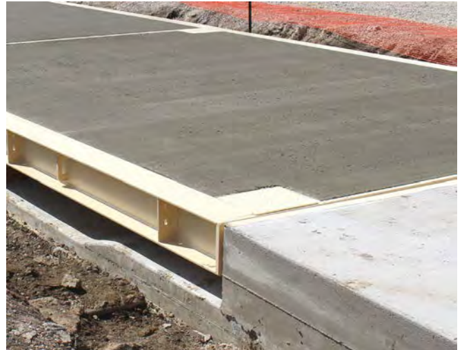
Apply a transverse texture to concrete with a wire broom (broom strokes perpendicular to the direction of traffic).
