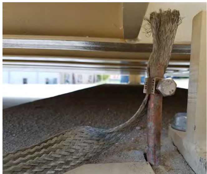
Ground Rod Connection
