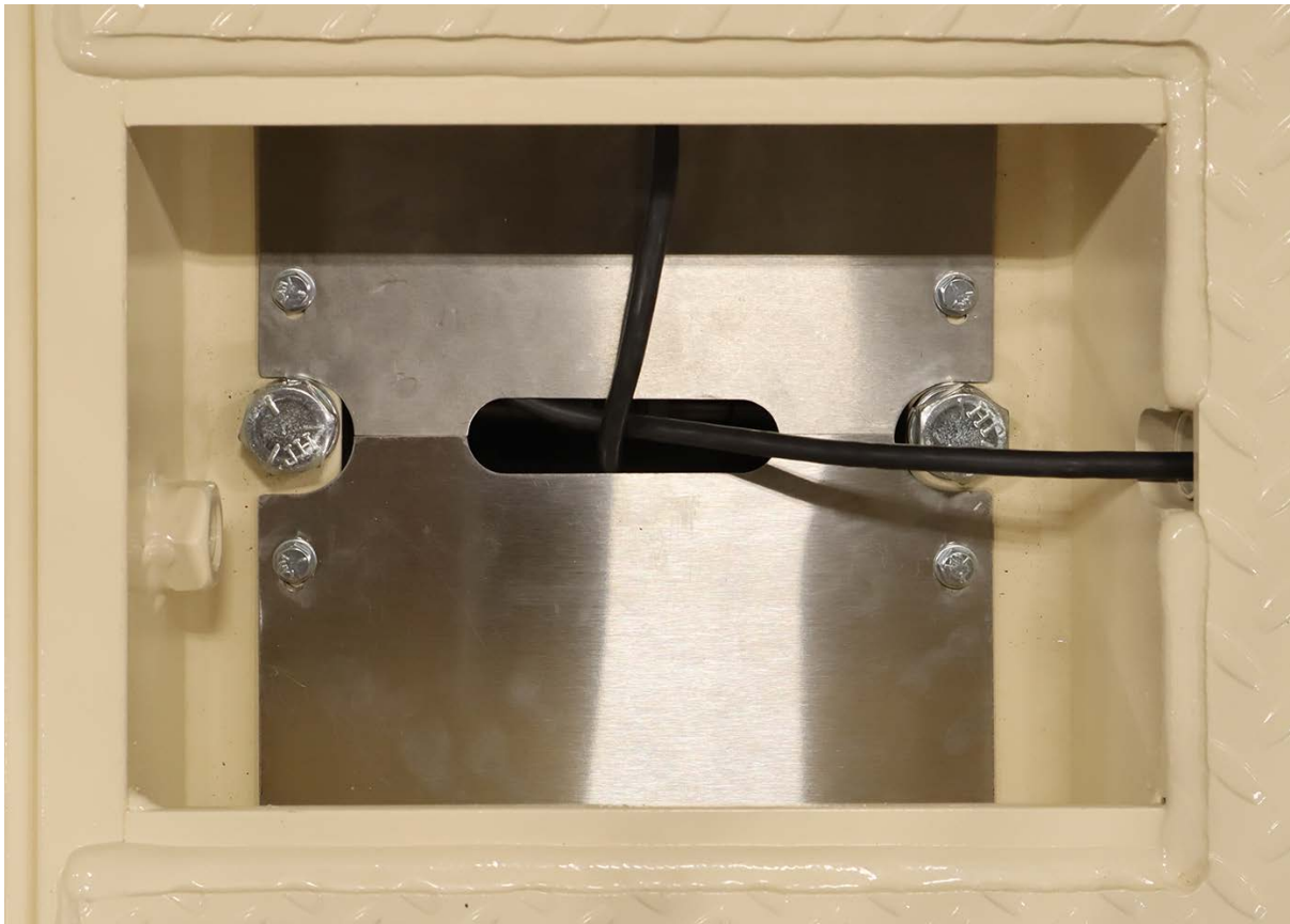
Installed Rodent Guard Shown
