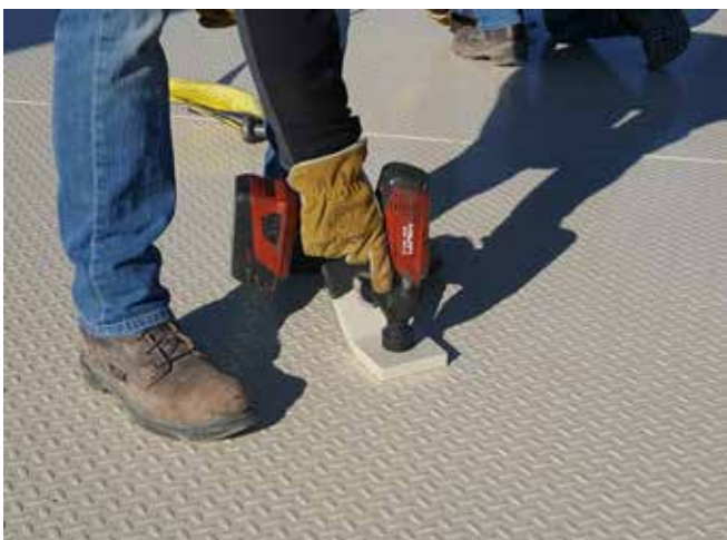
Remove lifting lugs from the first bridge module and install them on the second.
