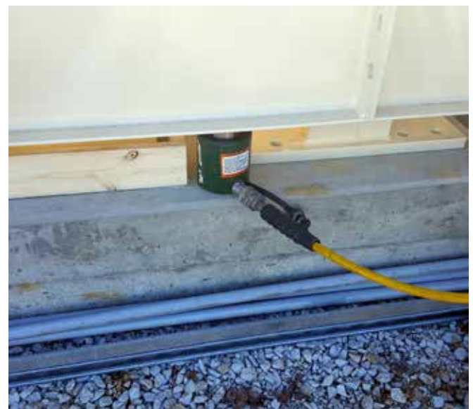
Lift bridge with a hydraulic jack, remove wood blocks, then lower onto load cell.
