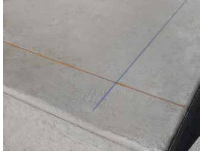
Per foundation drawing, snap a lateral chalk line for aligning grout plates.
