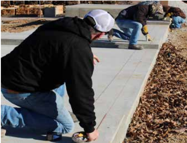
Snap a longitudinal chalk line on edge of piers per foundation drawing.
