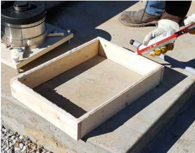
Use caulk on the form bottom to prevent grout from leaking underneath the form.
