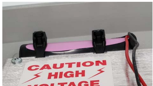
WRONG! Do Not Position Cable Ties Connection on Front of Batteries.
