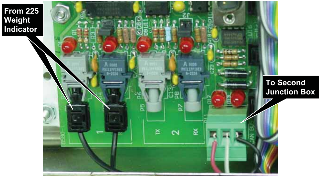
FIGURE NO. 23 CONNECTIONS FROM 225 TO FIRST JUNCTION BOX AND THEN TO SECOND JUNCTION BOX
